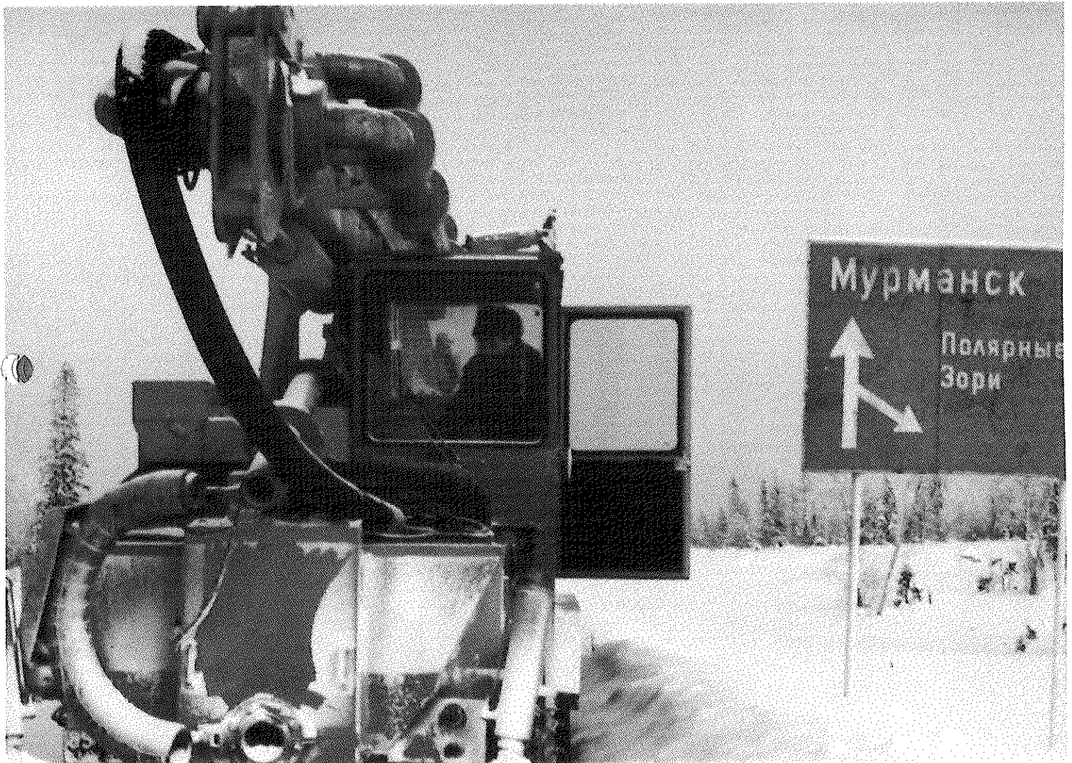
Worthington Pump's specially designed concrete pump is at home in the sub-zero temperatures north of the Arctic Circle.
